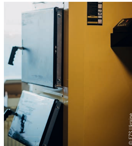
The new boiler installed in Hutsulshchyna National Park after the old one suffered catastrophic failure at the onset of winter.
